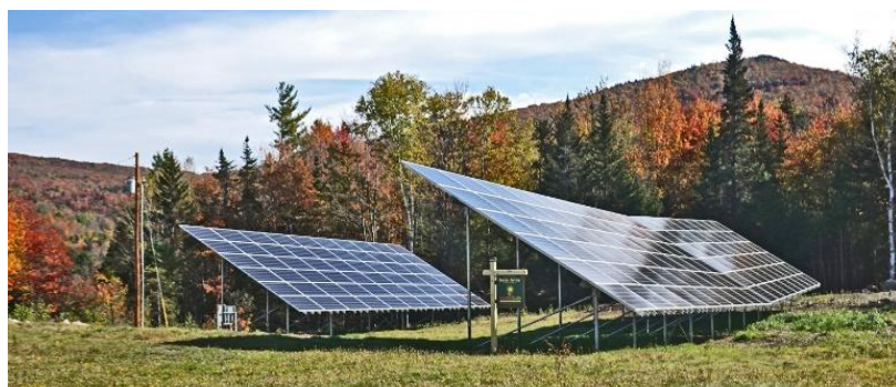
Solar Panels at Weston Priory
